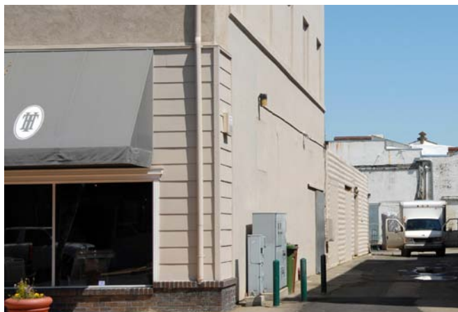
Utilities accessible along the side of buildings.
