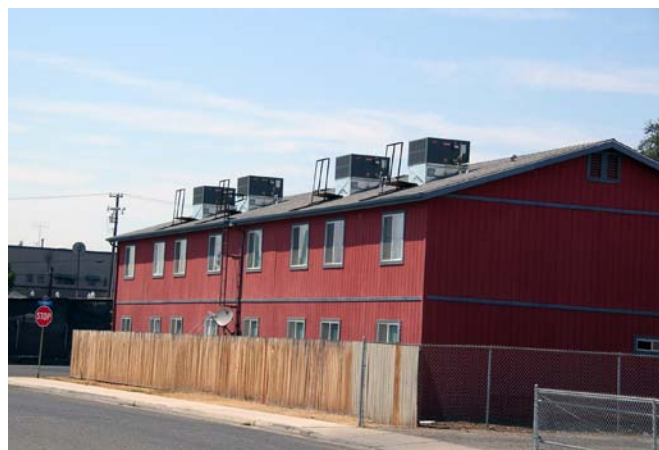
Rooftop mechanical equipment not appropriately screened.
